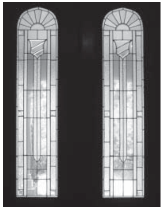
Entry hall windows at Seven Oaks, Bristol, R.I. (James Renwick, Jr., 1873). Photo: Astrid Liverman
